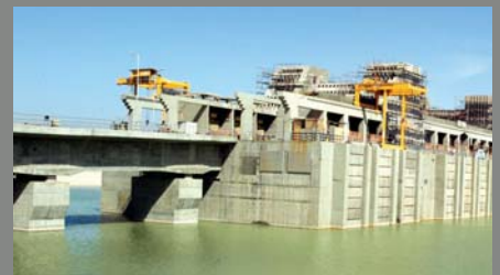
Mubarak Pump Station, Toshka
